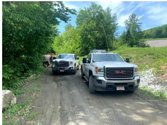
Monitoring well decommissioning setup along Copperas Road for former IC-01; looking south.
