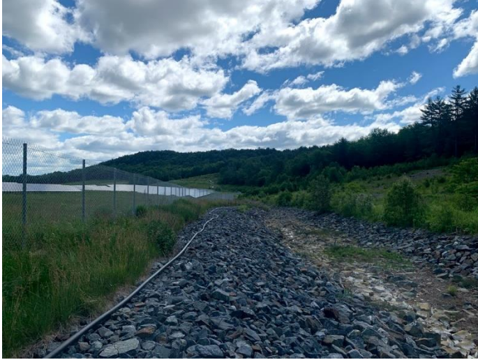
View of 2-inch poly conveyance line from water source pond; looking east along southern extent of TP-01.
