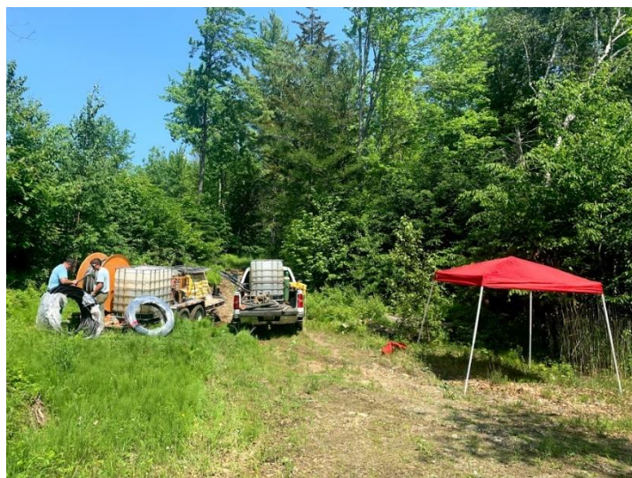
View of monitoring well decommissioning northwest of the former South Open Cut Pit Lake; looking west.
