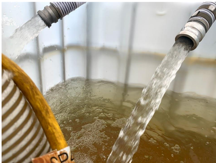
Discharge into the wet well during 1898 Adit dewatering activities.
