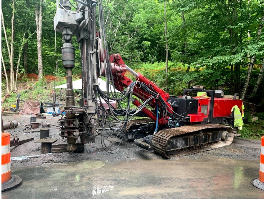
View of the drill rig setup along the west edge of Mine Road, ready to commence drilling at borehole PG-3.
