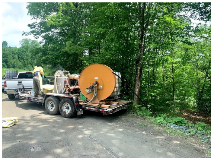
Monitoring well decommissioning setup along Copperas Road for former IC-01; looking northeast.
