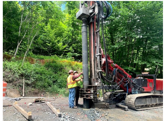
Checking plumbness during casing advancement of BPG-1; looking west-northwest from Mine Road / Copperas Road intersection.
