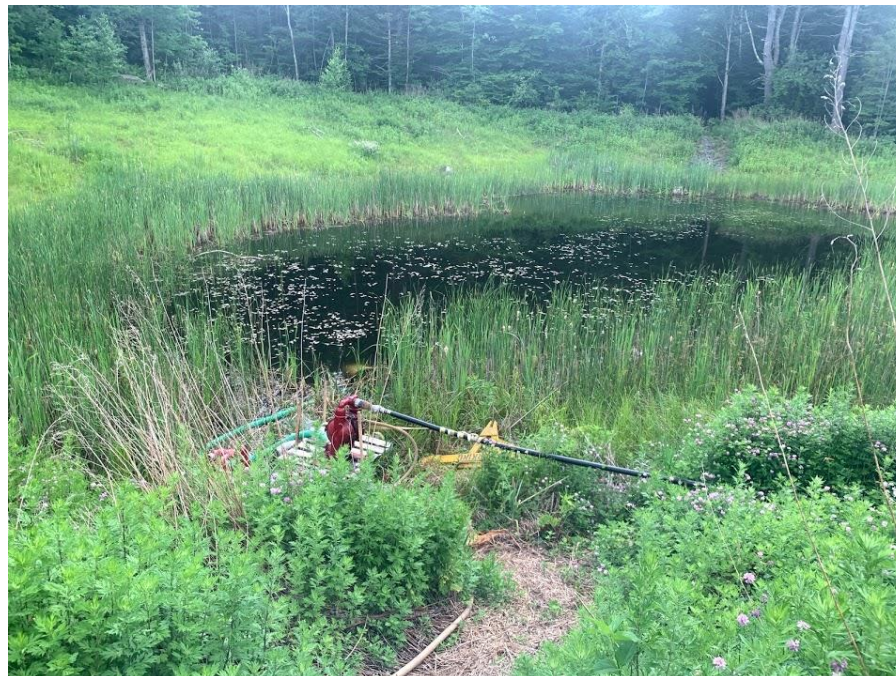
View of the intake hose, double diaphragm pump, and 2-inch poly water line at the water source pond.
