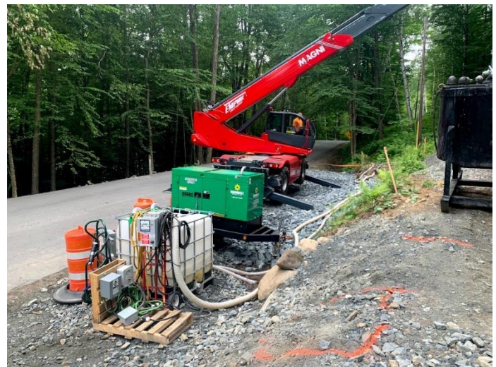
View of the relocated wet well and generator for the 1898 Adit discharge system; looking south-southwest from the Mine Road / Coppersas Road intersection.
