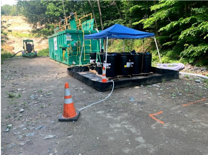
View of the dewatering pH adjustment system, frac tank, and high-head booster pump with North Open Cut visible in background; looking southwest.
